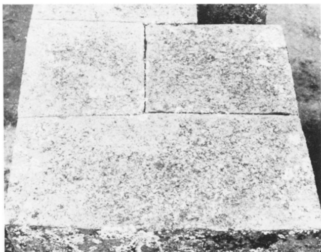
Fig. 34. Sometimes the building blocks were fitted carefully over the whole extent of the joining plane.
